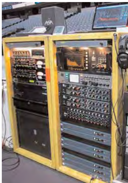
The two racks at front of house, topped by laptop with SMAART. Also note one of the first sightings of the new TC Electronic EQ Station, in the right rack under the dbx RTA-1.
