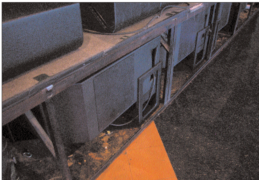
Four subs under the stage with special bracketing and space to breath.
