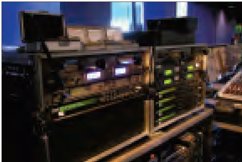
The primary monitoring setup ready to go, including Sennheiser "ear buds" on top of racks with Rane IEM processing.
