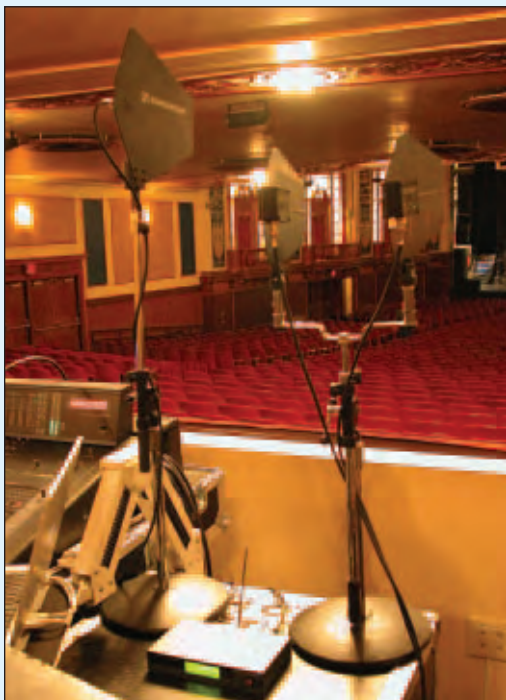
Wireless antennas stand-mounted at the mix position.
