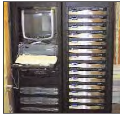
One of the system's "nerve centers" with MediaMatrix digital control/matrixing and plenty of Crown power.
